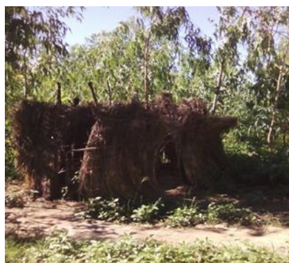
Picture 9: A makeshift urinal at Mhaju Primary School in Rumphi district in 2016.
